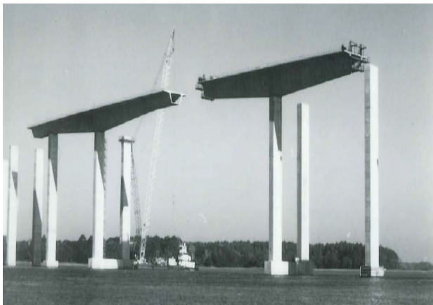
Shows the erection of the balanced cantilever portion of the James B. Edwards Bridge
