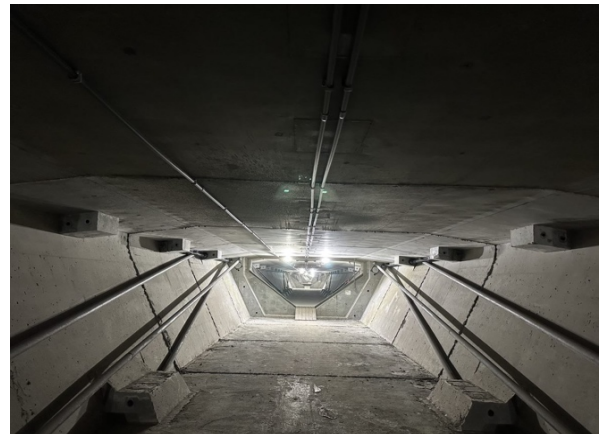
The interior of the box girder typical for the approach spans of the structures
