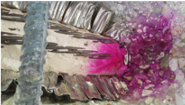
Figure 9: Field Carbonation Depth Testing at PT inspection Opening
