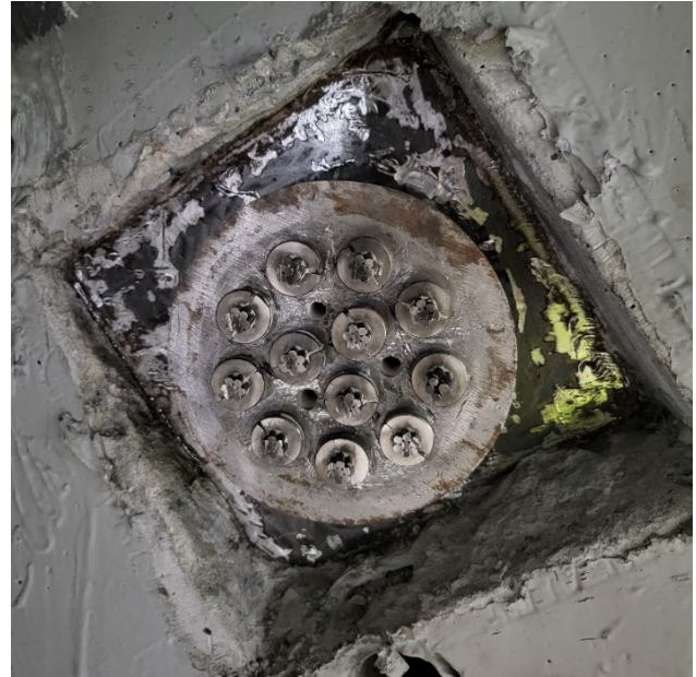
Figure 16: Grout cap and grout removed, with wedge plate and tendon tails cleaned and prepped for testing and PTI Impregnation
