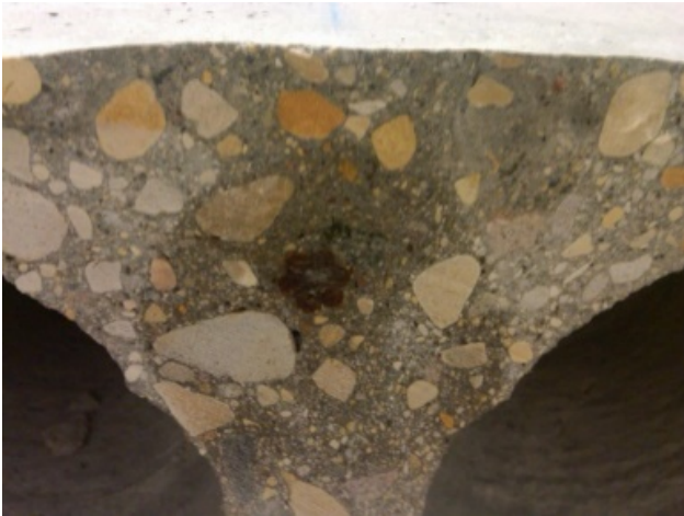
Figure 14: Concrete surrounding a single seven wire strand shows a radial pattern of Impregnation
