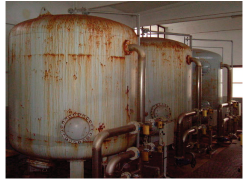
Condition of Tanks before ZincTape Application
