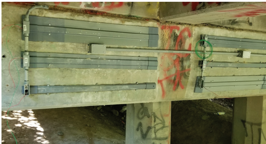
FIGURE 3 Surface-mounted distributed anode field study, Louisville, Kentucky.
